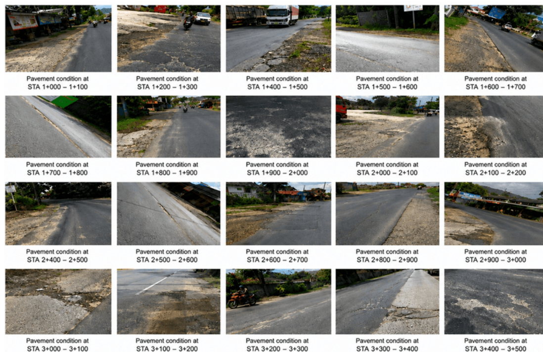
Figure 4. Representative pavement distress documented during the Pavement Condition Index (PCI) survey along the Ciganea-Cijantung road section (STA 1+000–STA 3+500)
